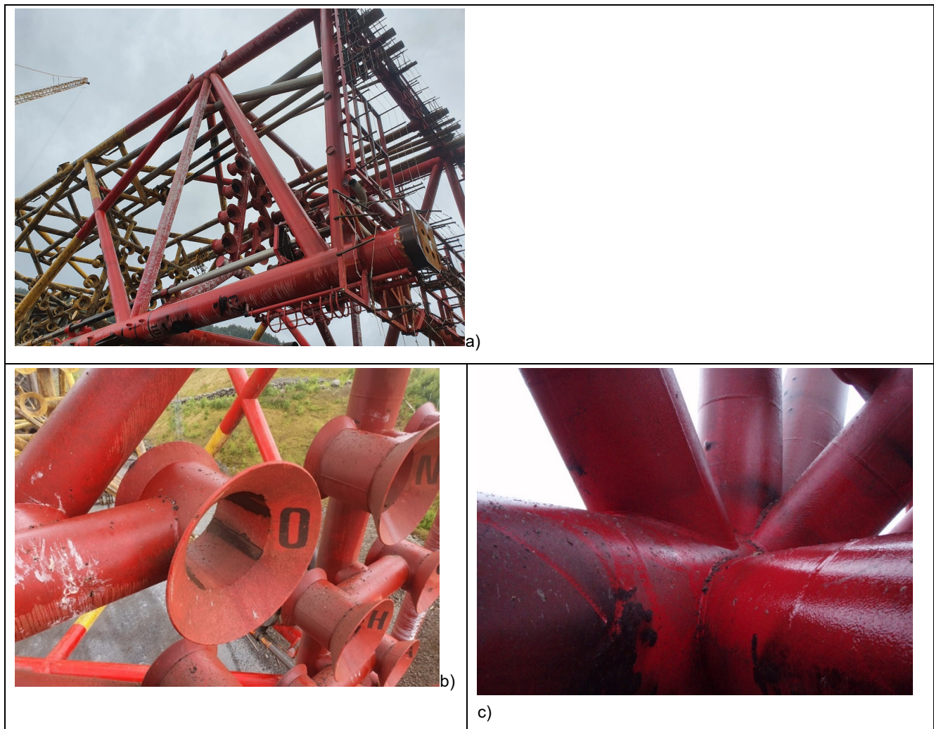
Figure 6-1 Coating appears generally good. a) overview Jotun B at the demolition yard b) conductor frame EL +8 c) node in splash zone, ref. /15/.
