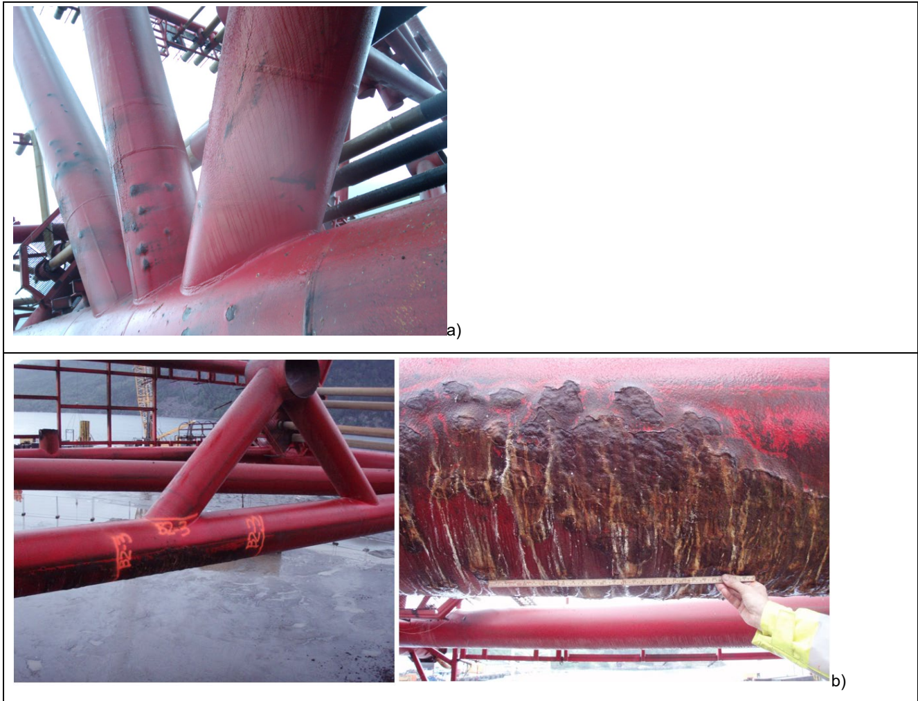
Figure 6-2 A few areas with coating damage at EL +8.5. b) Corroded area further examined with UT and up to 4mm wall thickness reduction was found, ref. /15/.
